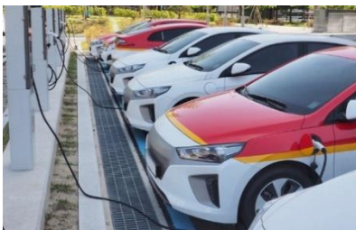
An example of a charging hub, credit: Western Power Distribution (WPS)
